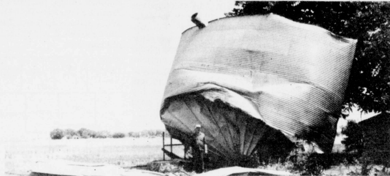
TORNADO DAMAGE —Herbert Jacob stands in front of a storage bin damaged by a small twister southeast of Winters.
