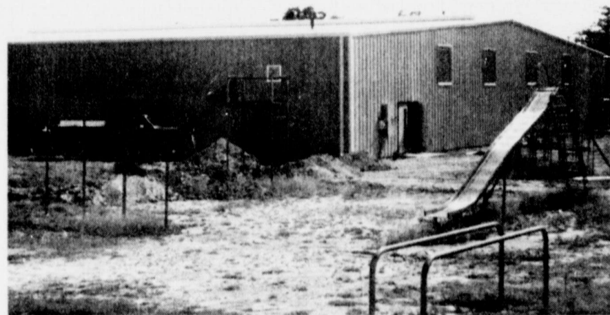
Ready or not, here we come! Work continues on the 12,000 sq. ft. building which will be used for classrooms for grades 2-6. The large metal structure is scheduled for completion in time for the first day of regular classes on Monday, August 26.
