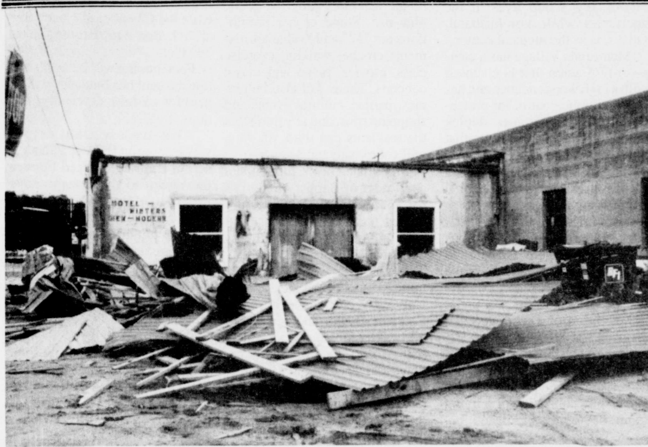
What's left of the roof of Winters Paint and Body Shop at the corner of Main and Wood Streets is pictured above. The roof was removed by high winds last Saturday night, damaging a corner of the building and leaving the roof in the middle of Wood Street. City street crews were called out to remove debris from several areas in the city.
