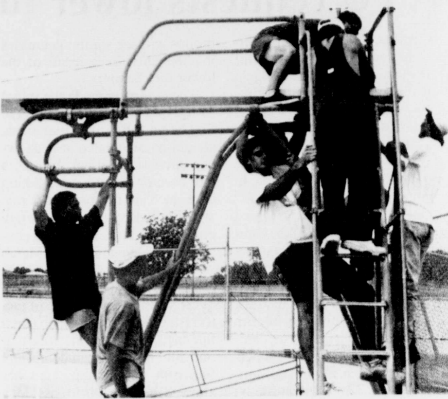
Highway department crew? Looks like it with two working and five hanging around, but they've really gotten most of the work done. Assisting in the installation of a new high diving board at the City Pool are, left to right, Bodie Collins, Josh Awalt, Dan Killough, Kelly Spill, Chris Matthews, T.J. Shields, and Brandon Killough.
