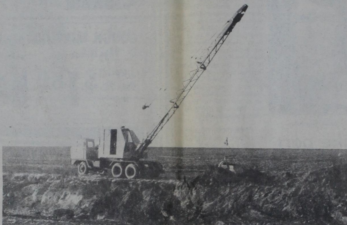
DIMMITT WELDING & ELECTRIC'S CRANE ON THE JOB ... Biggest machine around for excavating tailwater pits
