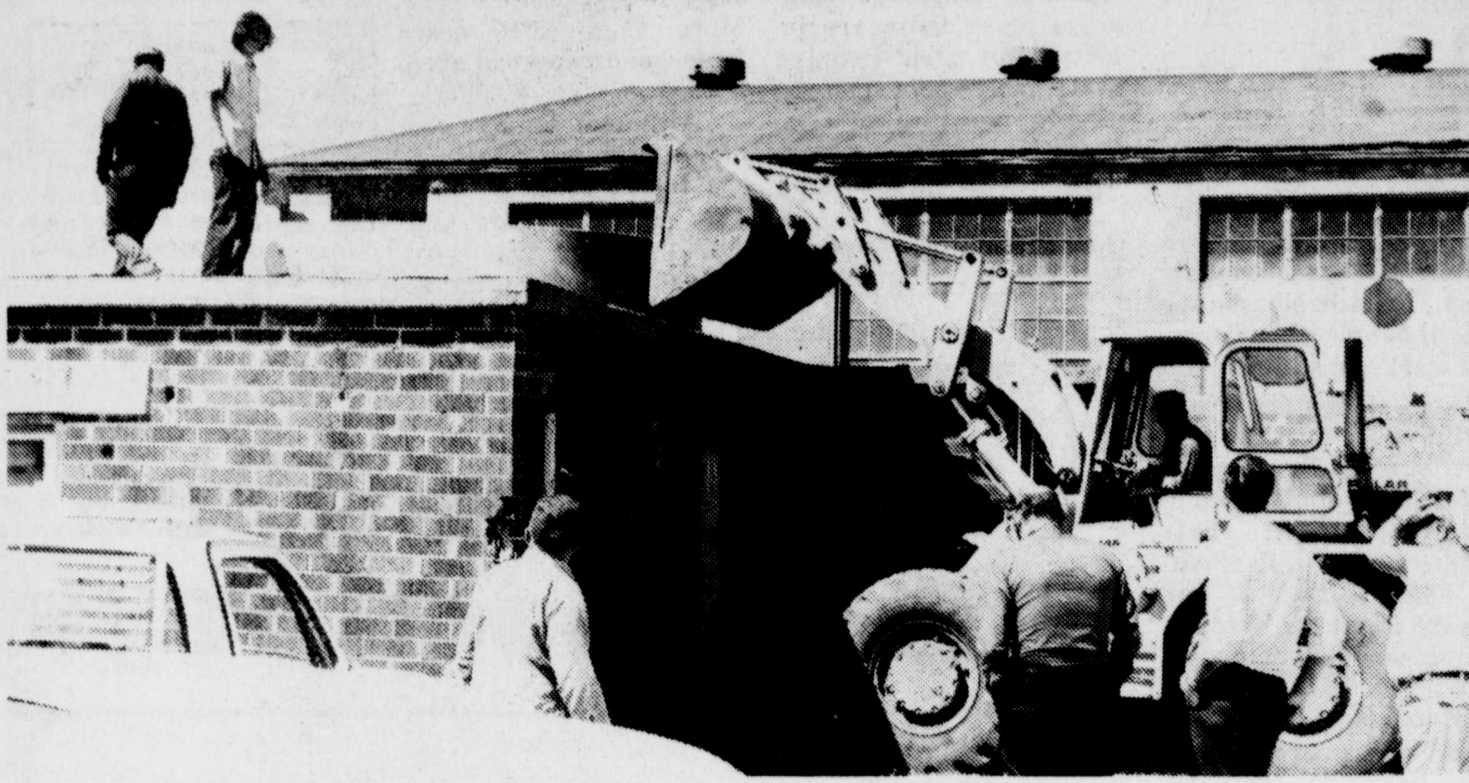
LAST OF THE PLANT—City crews prepare to remove a water tank from an outbuilding of the old City Light Plant, the last of the equipment remain-
