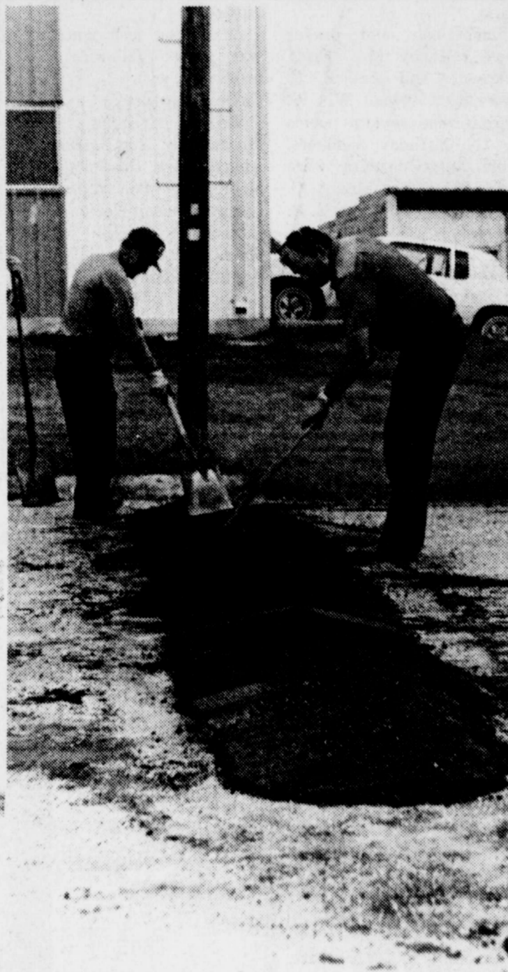
a speed breaker (bump) on a street near the school. This bump and others were installed Thursday of last week, and then removed the following day, because they were too high. City officials said lower breakers will be installed this week.
