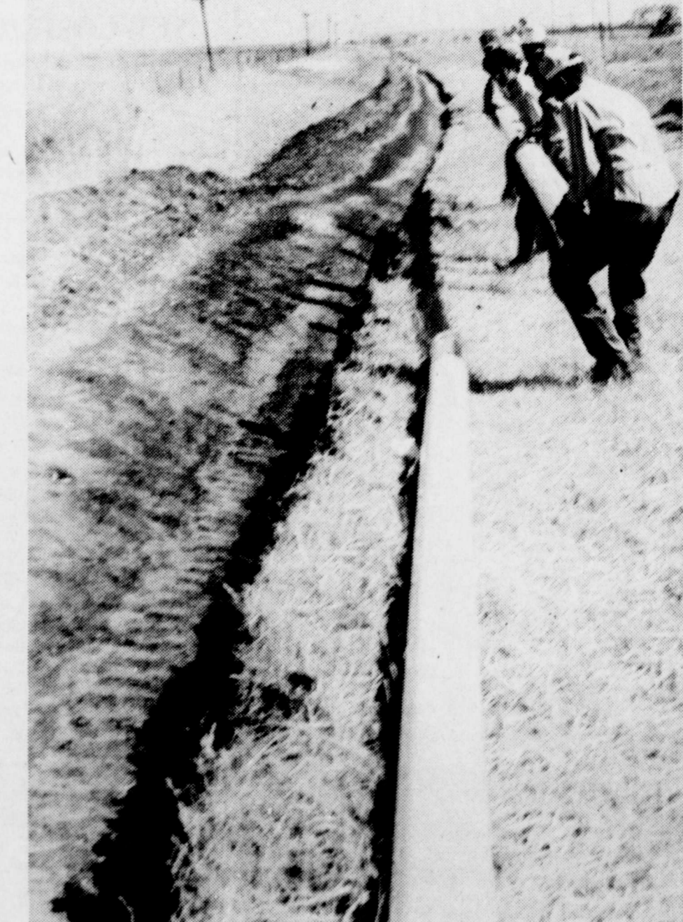
PIPELINE —Stringing of the PVC pipe from the three wells to the lake is a fast process, as only a shallow ditch is dug and the pipe connected with a plastic cement. The pipe was installed
