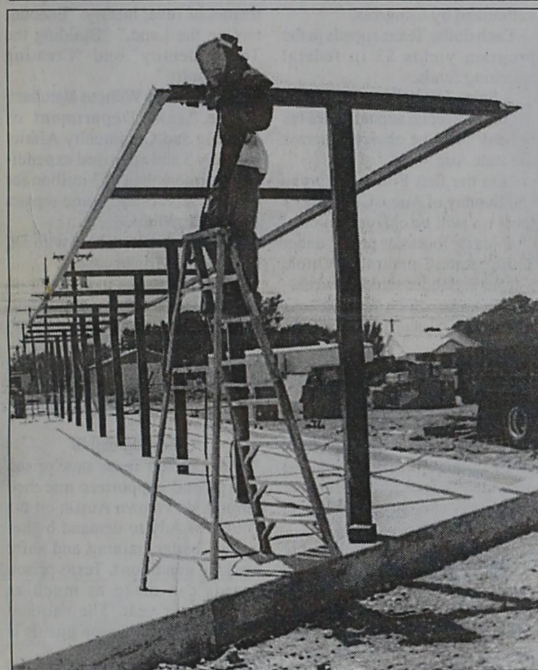
MAY I TAKE YOUR ORDER, PLEASE?—Brian Cuffey of Lampasas, an employee of Mira Enterprises, does some welding on the drive-up awning supports at the Sonic Drive-In in Dimmitt, which is scheduled for completion, hopefully, by the first part of August. Photo by Linda Maxwell
