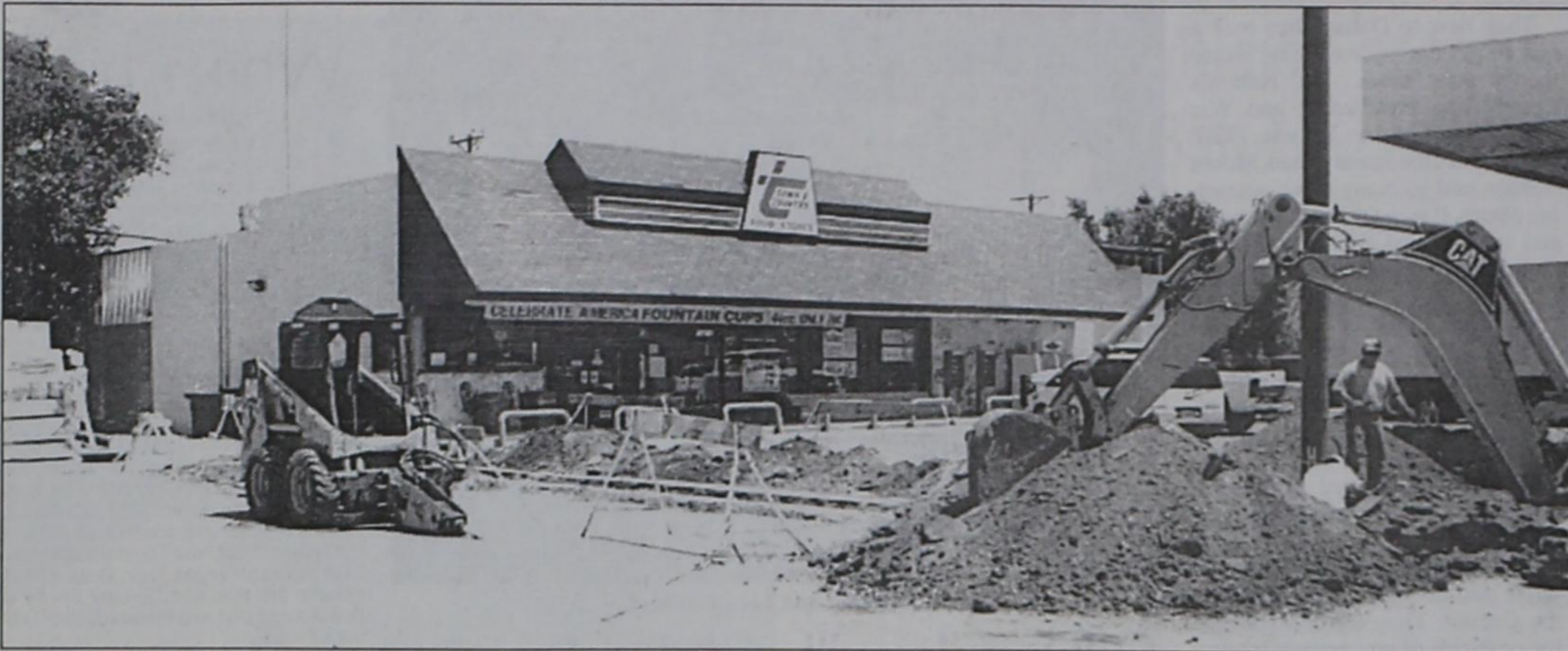
A "COUNTRY KITCHEN" eating establishment will be installed in the Town & Country Convenience Store in Dimmitt when construction is completed in a couple of months. The deli seating area will be enlarged and the entire store is being remodeled and given a "face lift," according to Dulia Perez, an employee of the local store. Gary Davis of San Angelo, construction supervisor, said his crew will be adding a 15 x 40-foot extension on the south end of the building and a 15 x 41-foot extension on the northeast corner of the building. He said they also will be extending the canopy and adding another gas island for fuel customers. Although access may be a little bit difficult, they are still open for business.
