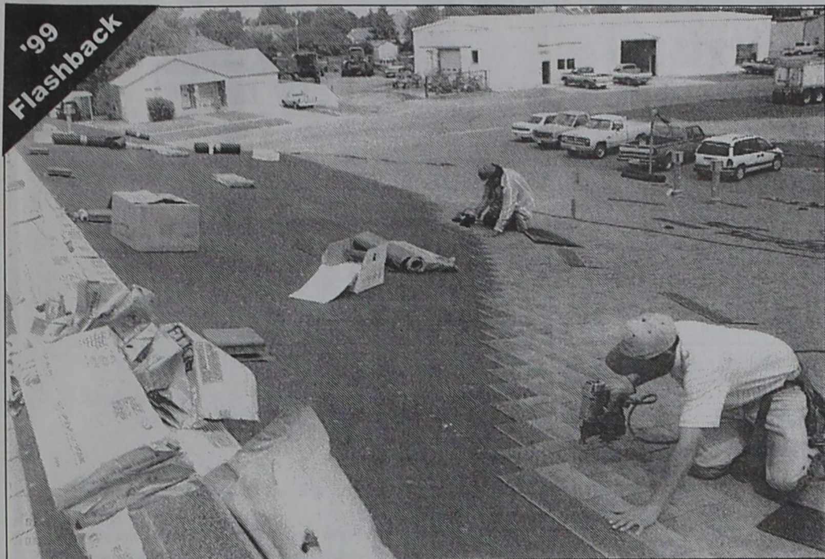
A FAMILIAR SIGHT throughout the county this year was this one, of roofers working from dawn 'til dusk to repair hail damage on hundreds of homes and businesses. Here, Jesus Miramontes (foreground) of Littlefield and Marco Zarate of
