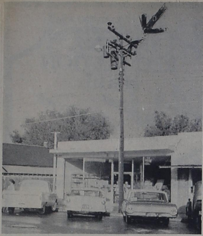
ELECTRIC SHORT -- The arrow in upper right points to a strip of tar roofing paper which wrapped around electric lines here during Thursday afternoon's storm causing power to be off in some areas of town. Similar debris, which came from the roof of Parmer County Farm Supply building, is shown on the street in the foreground.
