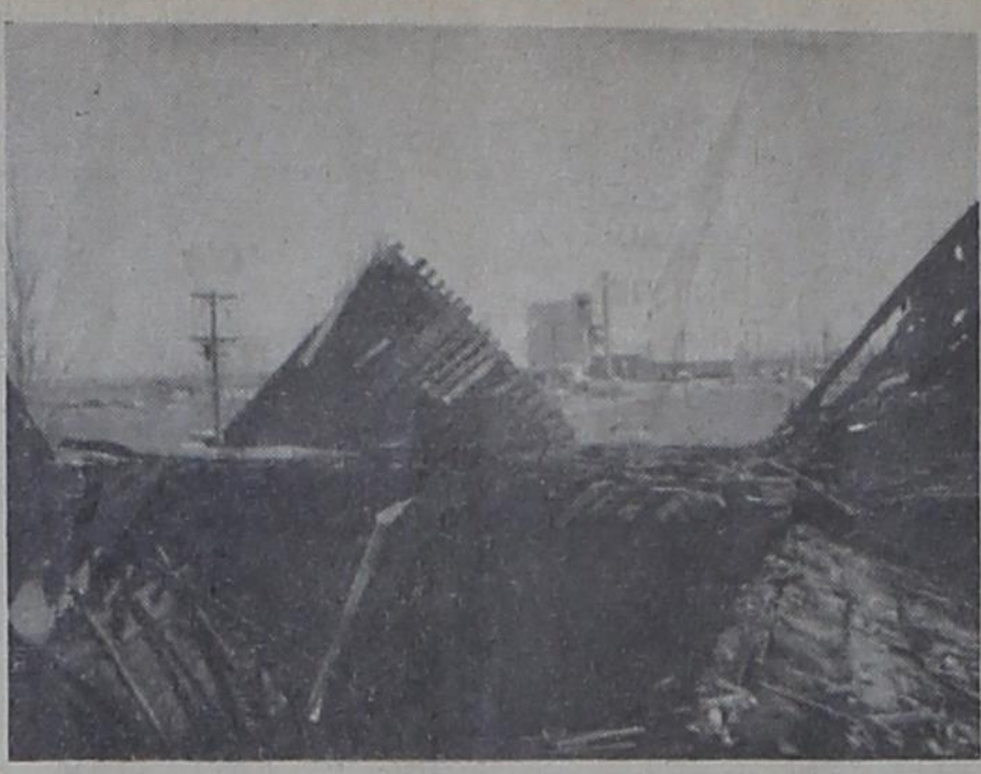
ONCE THE MAIN ROOM of the XIT ranch house, this room has been almost filled with roof timbers and shingles that caved in when the roof gave way.
