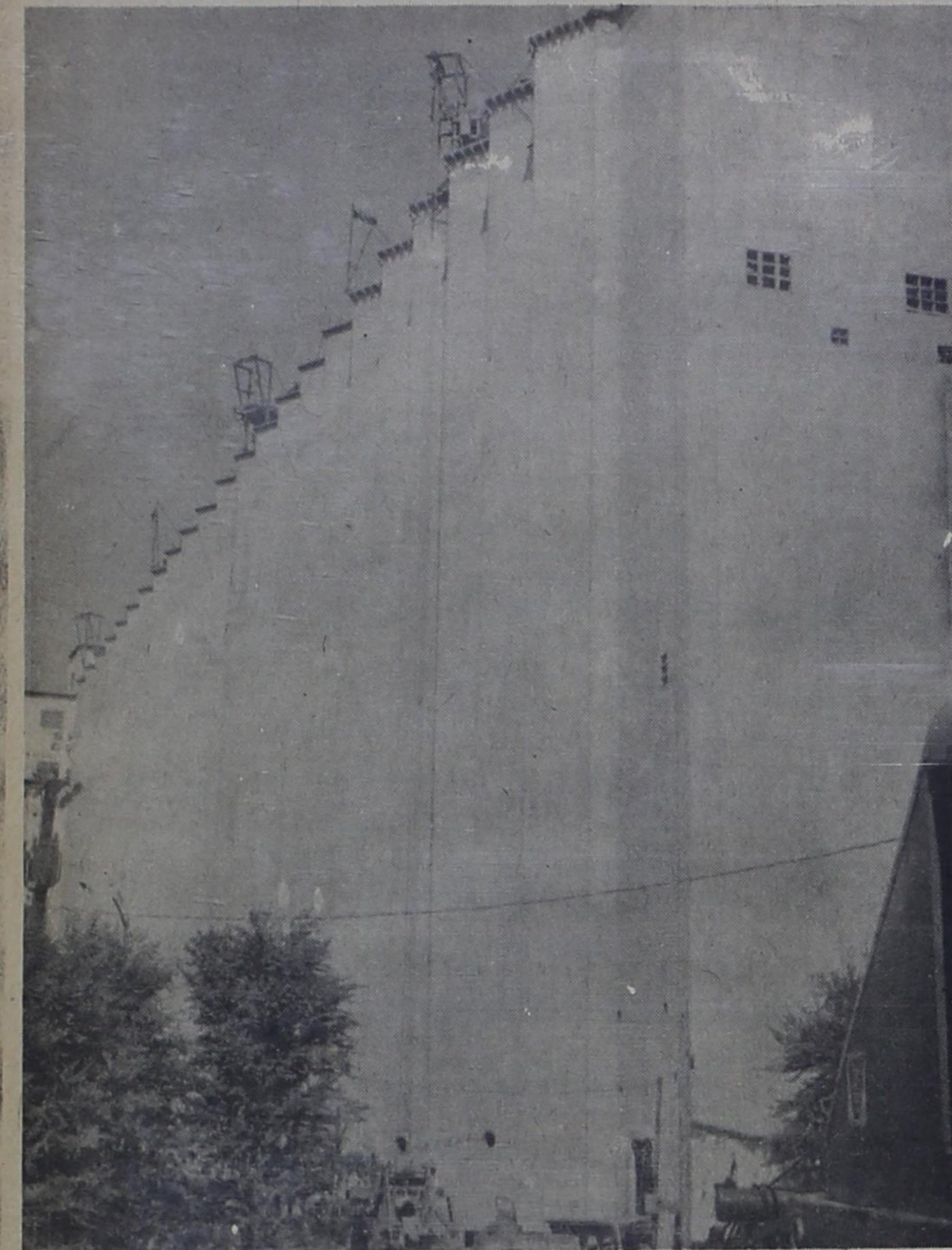
SOON TO BE COMPLETED is this 1 1/2 million bushel storage addition at Sherley Grain Company in Bovina. This is one of the latest elevator construction projects to be undertaken in Parmer County. In all, the county has a grain storage capacity of 35 million bushels.
