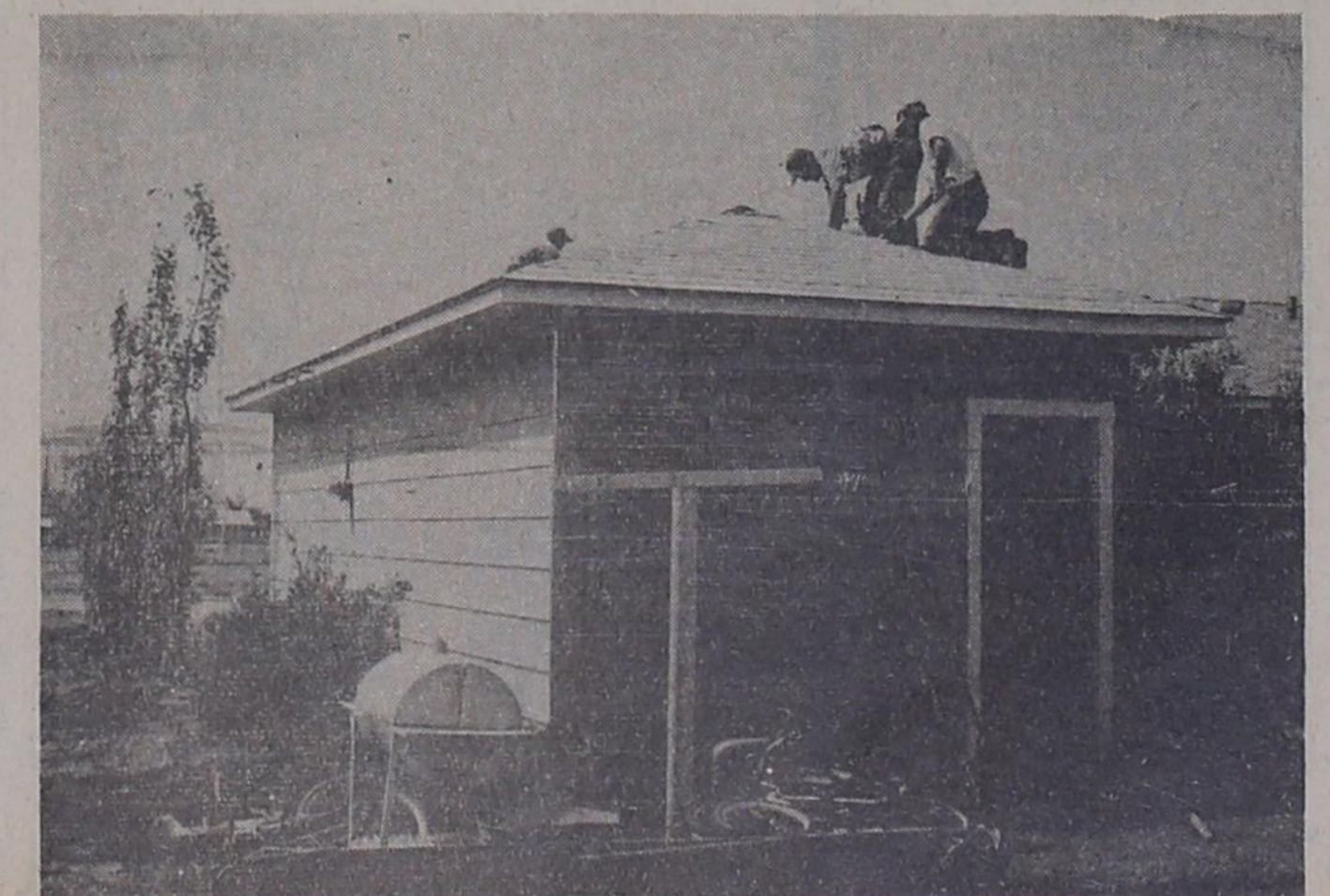
ROOF REPAIRS--Hail damage to roofs was still being repaired this week. The above crew is repairing the roof on the Hutto home at 605 Ave. G.
