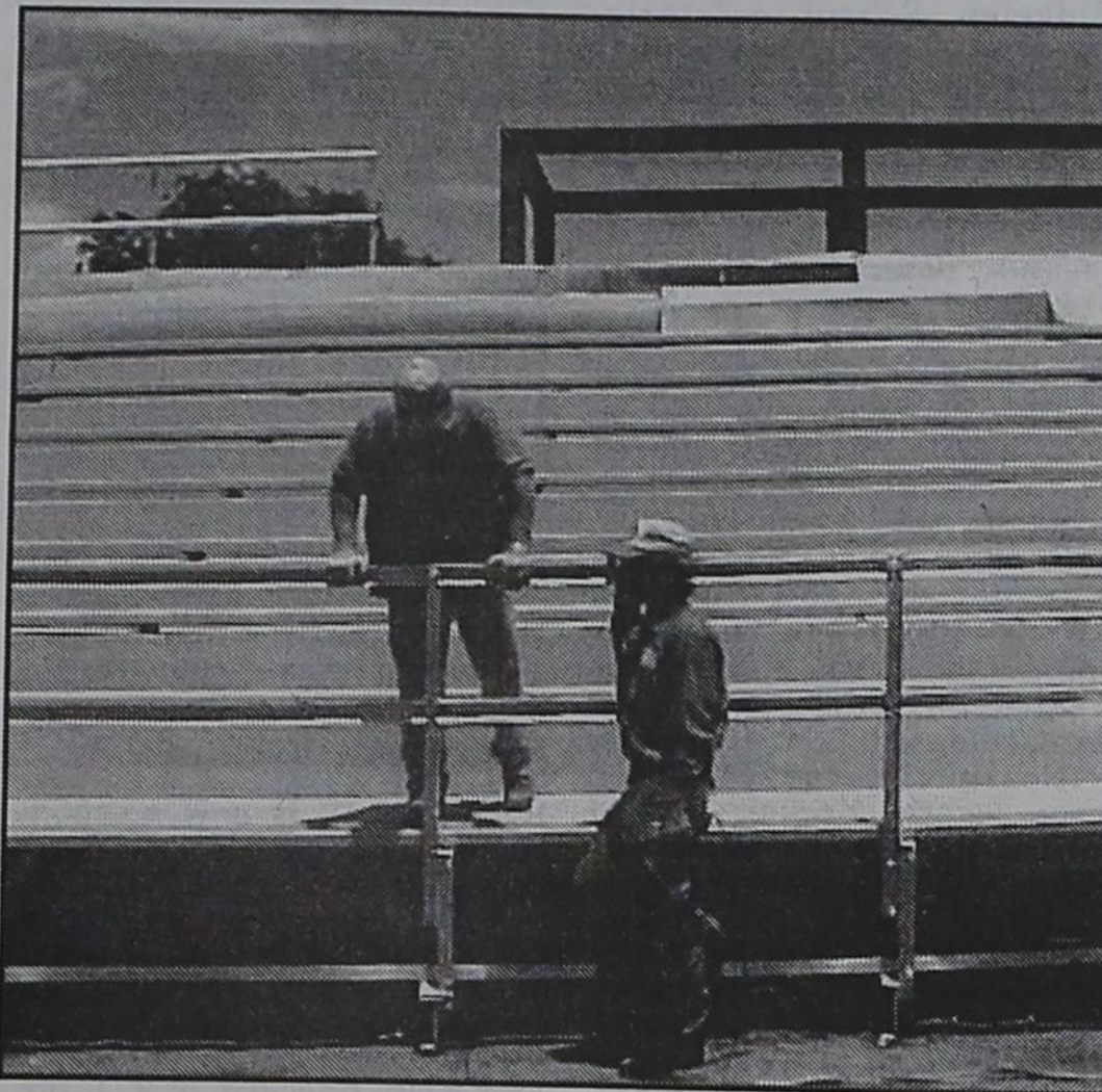
HOT WORK... The football stands were a hot place to work last Tuesday as temperatures reaches 98. Kevin Eschberger, left, and Stan Miller were finalizing construction in spite of the heat. Eschberger is the new ag teacher at BHS.
