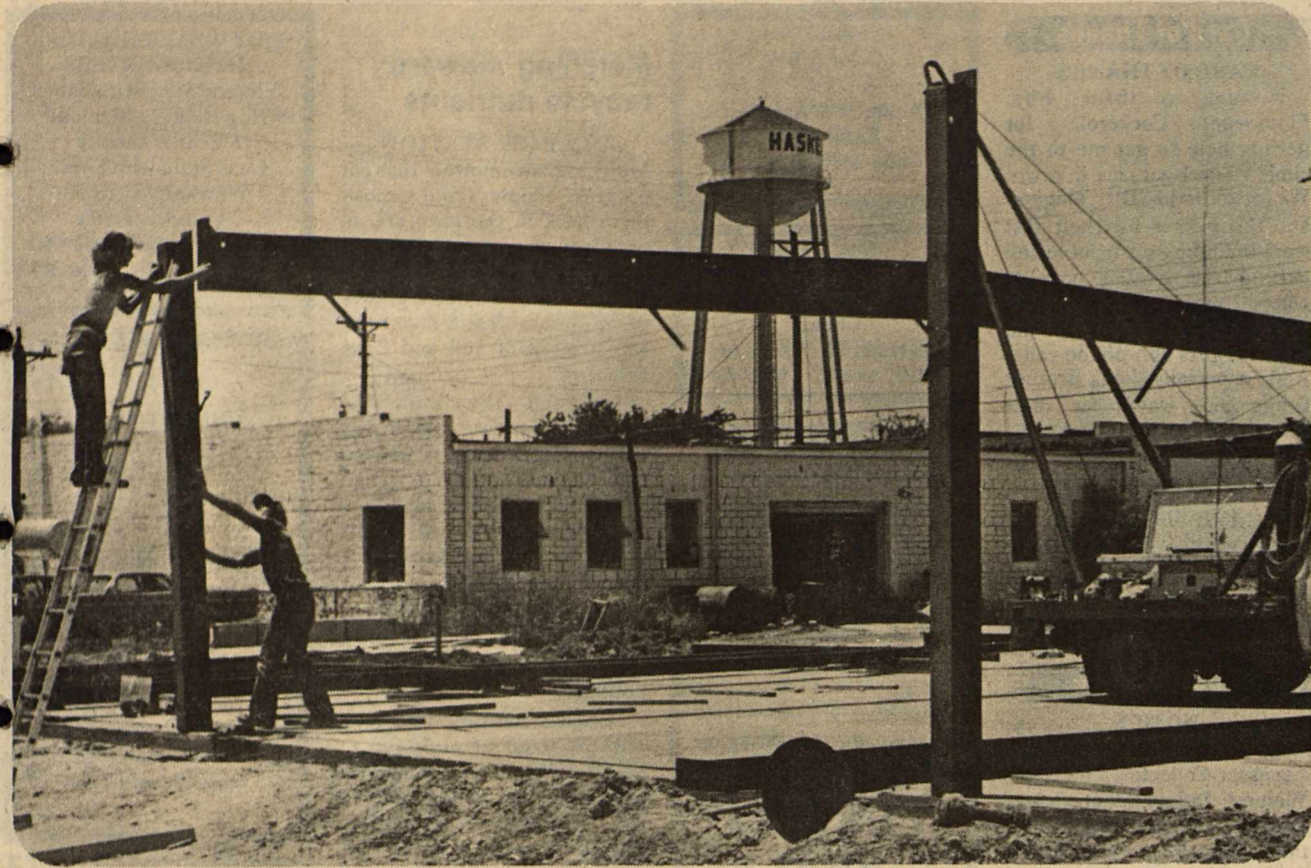
SUPPORT BEAMS were placed in position on the new Fire Station Monday and Tuesday and work on wall panels was started Wednesday morning. Workers expect to complete the exterior of the building by the
