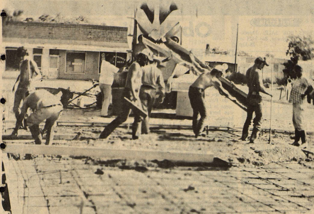
THE FIRST LOAD -The first load of concrete was poured for the slab of the new fire station Tuesday morning. It will take around 110 yards of concrete for the footing and slab. The entire slab should be completed today. The building material
