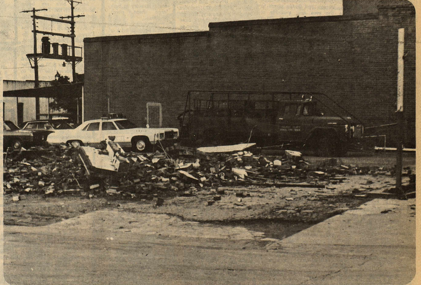
A SMALL PILE OF BRICKS is all that remains of a vacant gas station which recently occupied the future site of a new fire station in Haskell. Members of the department have almost completed the removal of the gas station and are hopeful that foundation work can be started in the
