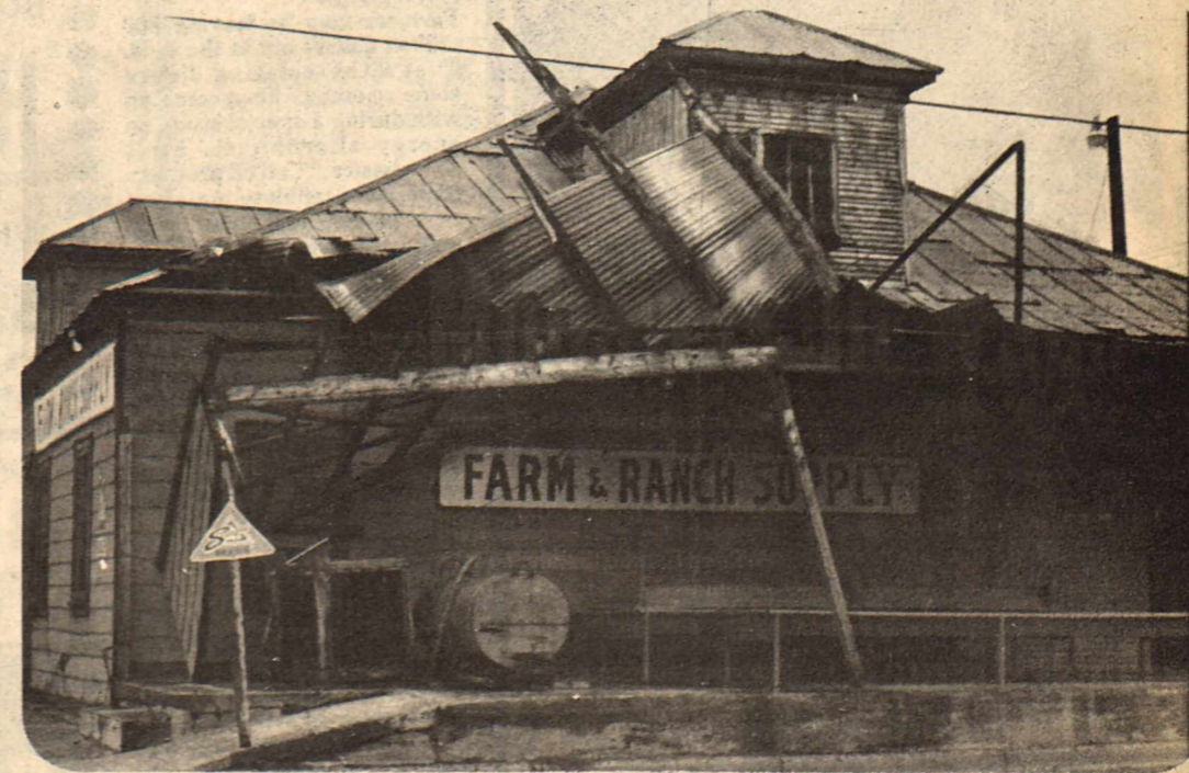
THE WINDS CAME...and then came the rain...High winds left this damaged building in its wake Monday afternoon, however along with the wind there followed some rain of varied amounts throughout Haskell County. Reports ranged from a sprinkle to a down pour depending where you happened to be. On checking with Pete Beecher of NCTMWA he reported that there was no noticeable rain in an area that would effect the Miller Creek Lake. (Staff Photo)
