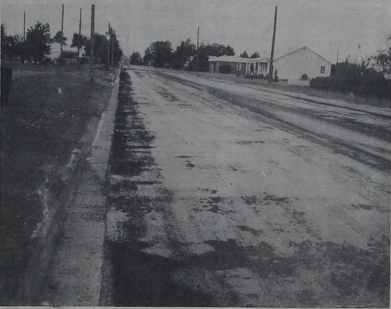
STREET IMPROVEMENT WORK --- Work on paving 12 additional blocks of Bovina streets is underway. Curbs and gutters have been finished with the paving itself the part that remains to be done. Caliche base is being rolled and packed at top. The lower scene shows a street covered with oil in preparation for the asphalt. Contractor for the project is Jake Diehl Dirt and Paving of Muleshoe and Hereford.
