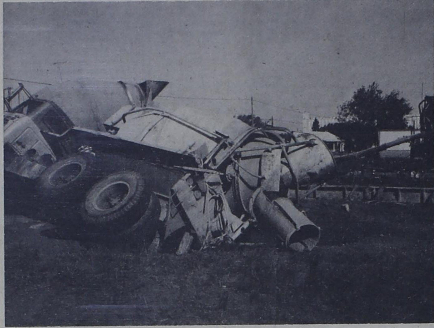
DIFFICULTIES --- An old septic tank or cesspool was responsible for a cement truck's sinking into the ground Tuesday morning in the 400 block of Ave. G. Work was beginning on a new home for the Isidoro Saldana family.
