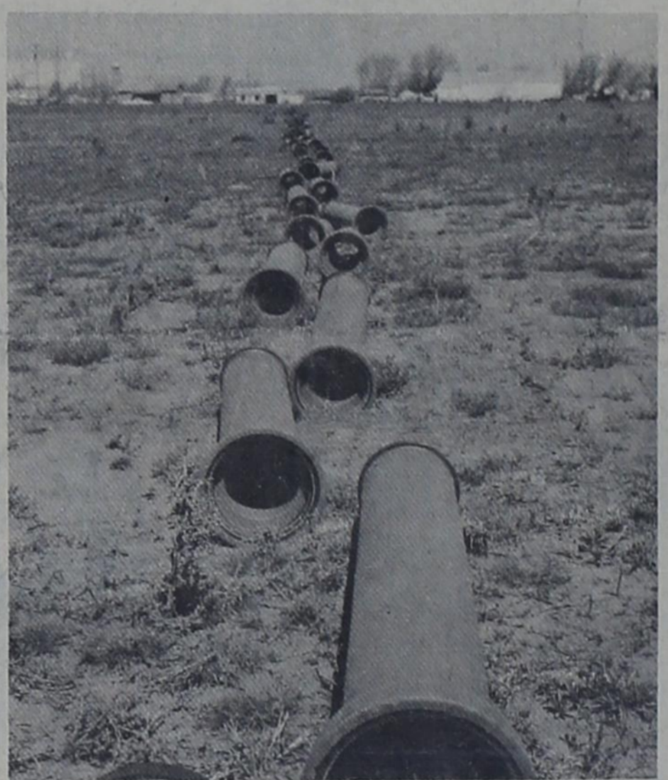
EXPANSION BEGINS --- Tile is on the ground in Eastview Addition in preparation to installing water and sewer lines there. Jones Construction Co. of Big Springs was awarded the contract by city council Wednesday.
