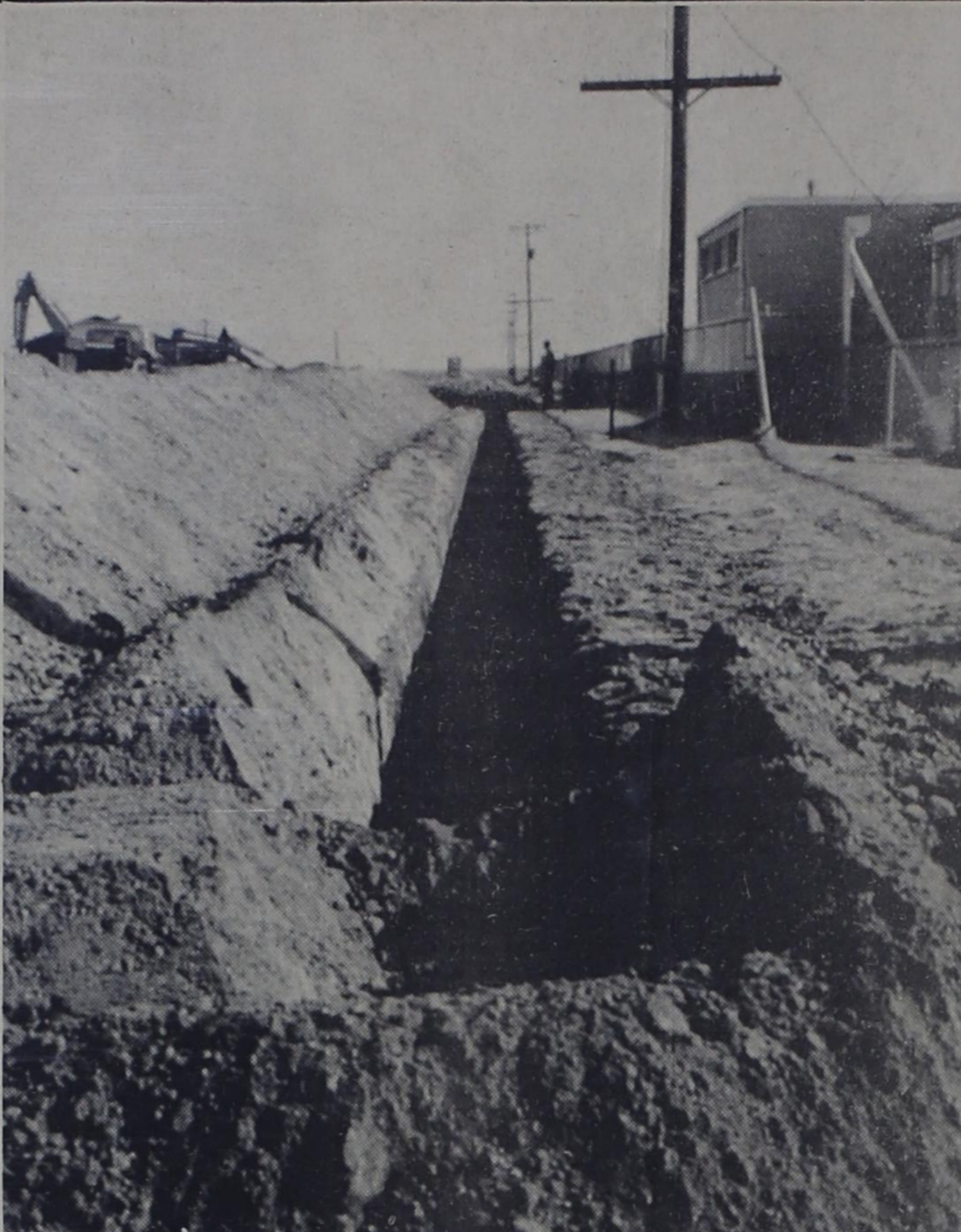
NEW SEWER LINE -- City of Bovina this week is extending the city sewer line in Ridgelea Addition and also tunneling under Highway 86 to connect with school property where the proposed new elementary school will be constructed. The line also runs behind Ridgelea Drive to provide service to new homes now under construction. The extension will connect with the lift station to the southeast.
