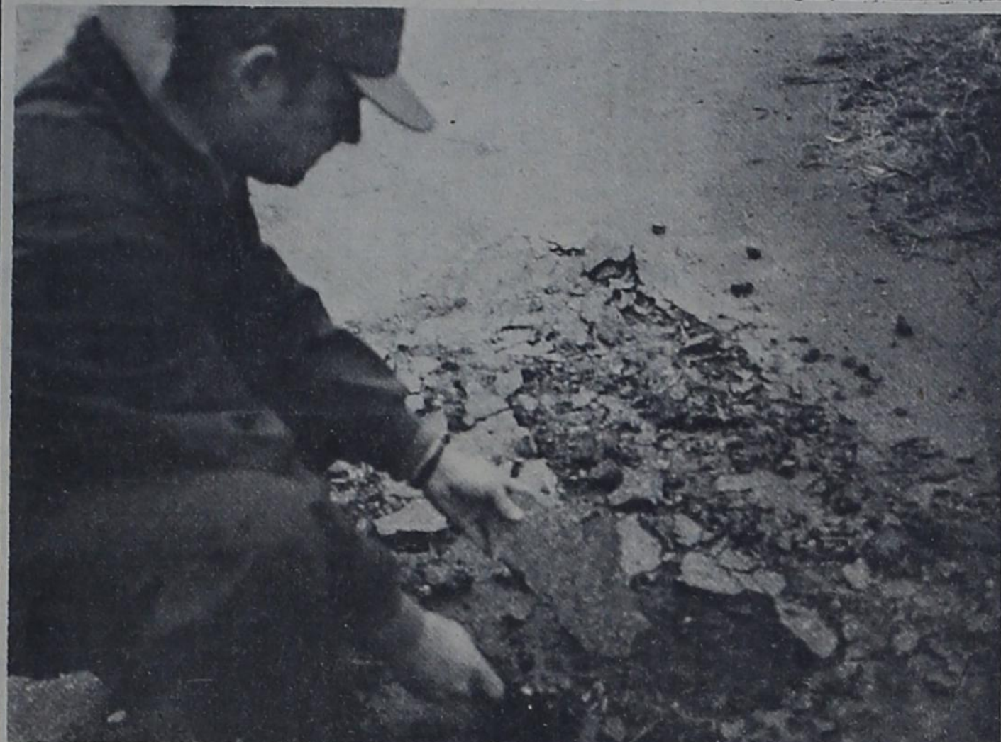
AFTERMATH --- Darrell Read, City of Bovina water superintendent, looks over the pavement damage caused by snow and ice that stayed on the ground two weeks. City employees have already filled in many chug holes. Read says they will wait to repair other damage until moisture dries out.
