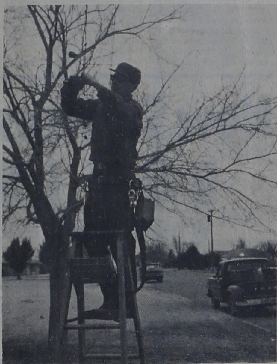
YULE LIGHTS -- Lewis McDaniel of Southwestern Public Service made electrical connections Monday at Bovina's city park in preparation for turning on Christmas lights this season. The lights had previously been strung by city personnel. Also being planned is a star to enlarge the decorations this year.
