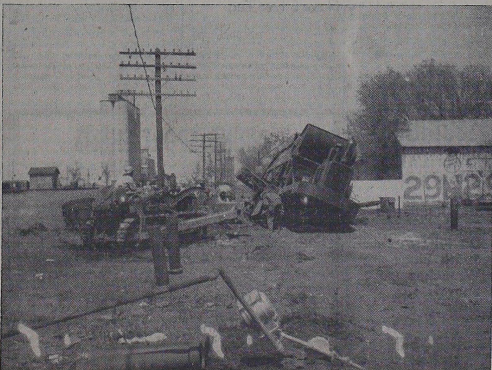
BIG MACHINE IN A HOLE—The giant trenchliner, which is being used to dig the ditches for Bovina's sewer system, almost turned over when it fell in a cesspool in the alley between North Street and the railroad. The machine at the left is being used to get the trenchliner "back on its feet." The picture was made Monday.
