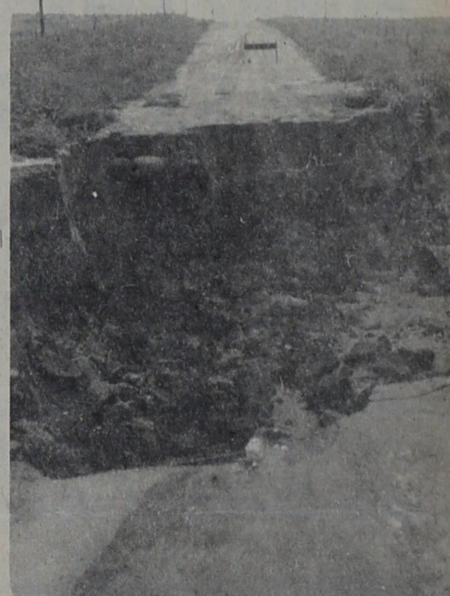
FLOOD WATERS WASHED OUT this road north of the Pleasant Hill community near Frío Draw. The washed-out area was about 15 feet in depth and 30 feet across. This area received nearly 10 inches of rain in one 24-hour period.
