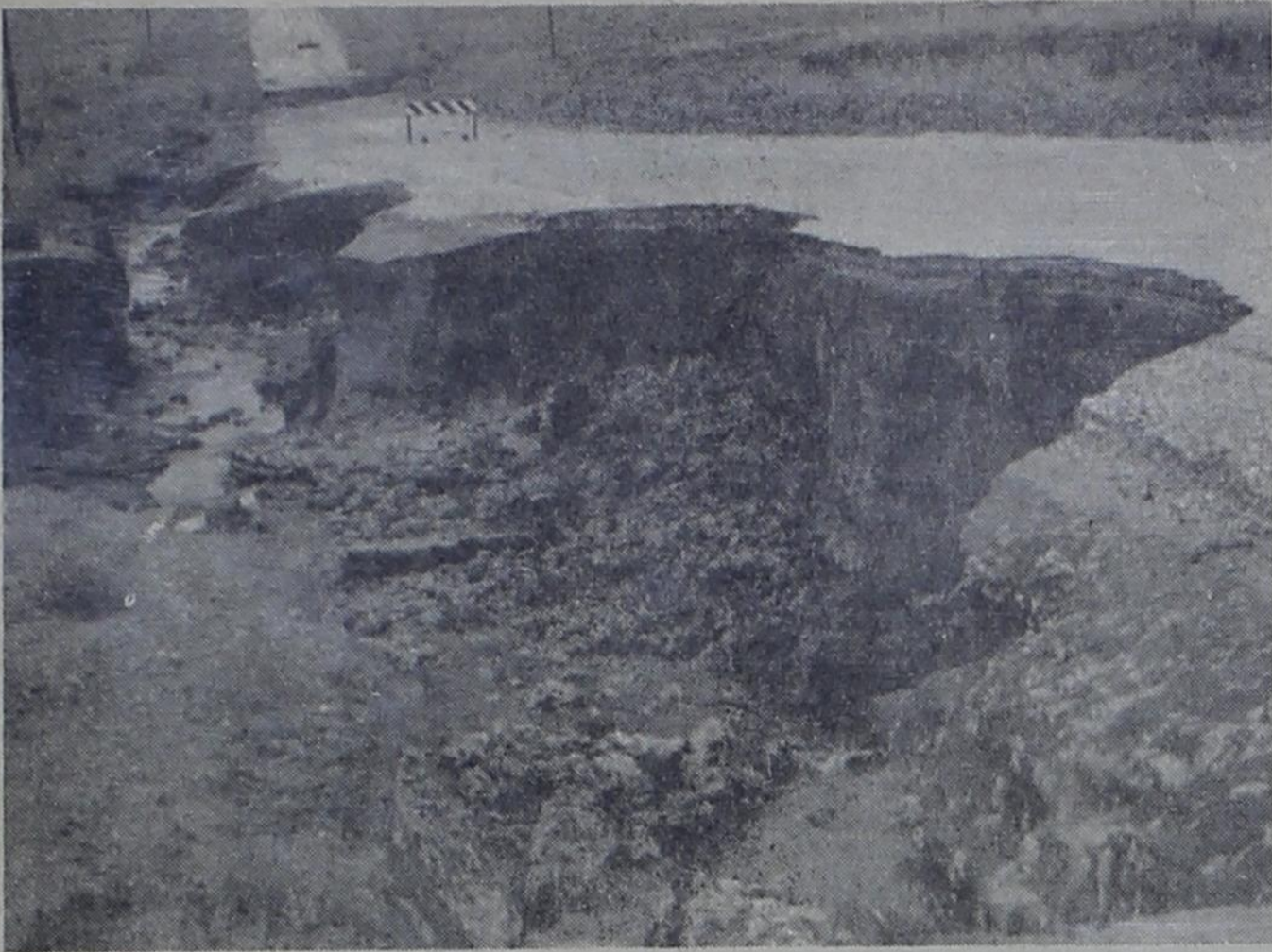
PART OF PAVED STATE LINE ROAD north of Pleasant Hill was washed away during the downpour. Further down the road (just off the pavement) is where the complete road was washed away. Beyond the next hill is Frio Draw.
