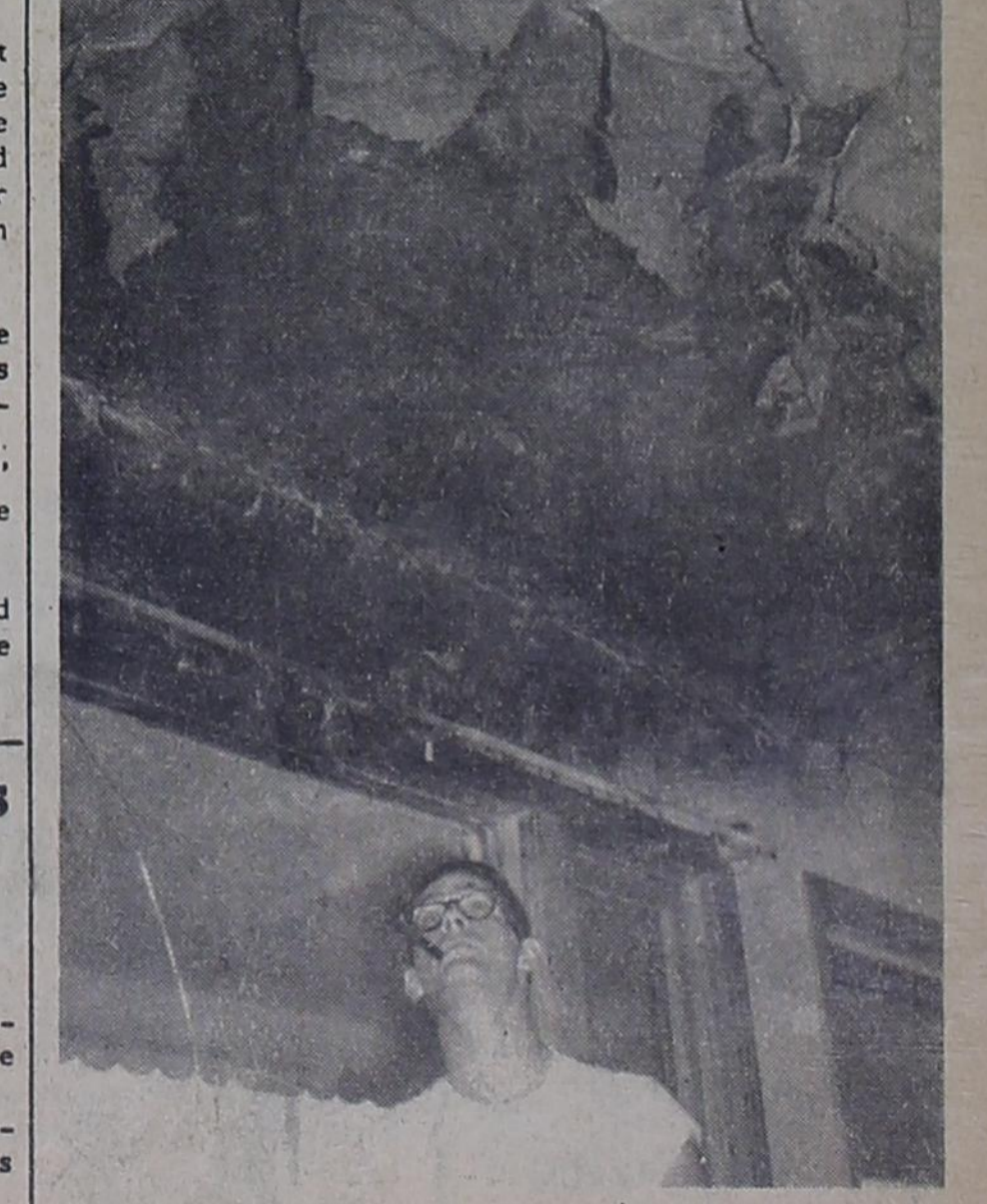
WAS SPREADING FAST--Max Gilreath, 18-year-old son of Mr. and Mrs. Boyd Gilreath, examines damage to ceiling in his home. The blaze climbed from a television antenna cord to drapes the window and onto the ceiling.
