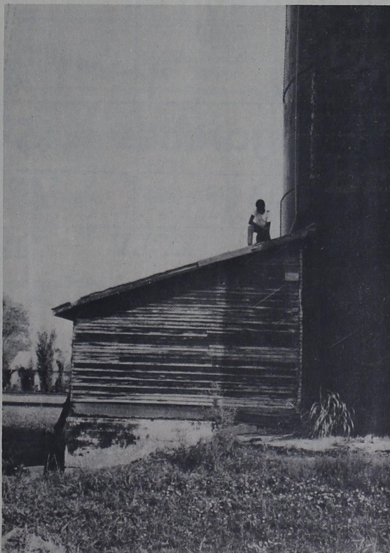
REPLACEMENT TIME --- This wooden structure, which for many years housed a city well pumping mechanism north of the railroad, has been torn down and will be replaced by a tile building. At right is a water storage tank. The improvement is being made to better protect the pump. Sherrill Lumber Co. has the contract for constructing the tile building. A top the building is Luther Robinson, who assisted in tearing it down.
