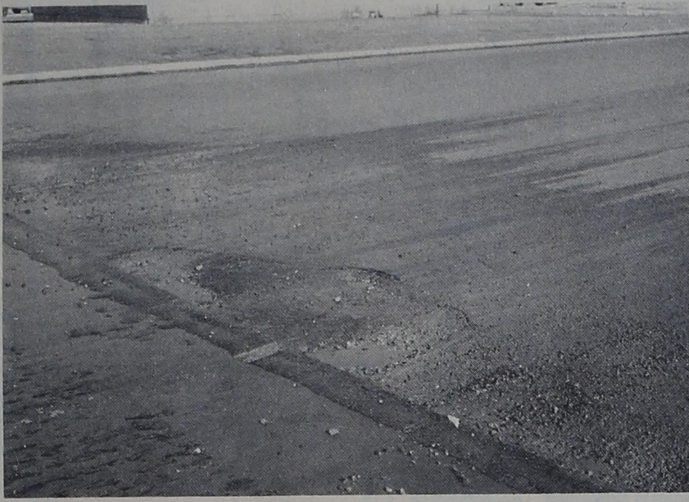
SNOW HAZARD --One of the disadvantages of snow is shown here in the form of a hole in city pavement. This chughole, which offers a jarring effect when struck by the front wheels of an automobile, is at the intersection of Third Street and Avenue D. There are other such blotches in city paving which have been caused by the snow.
