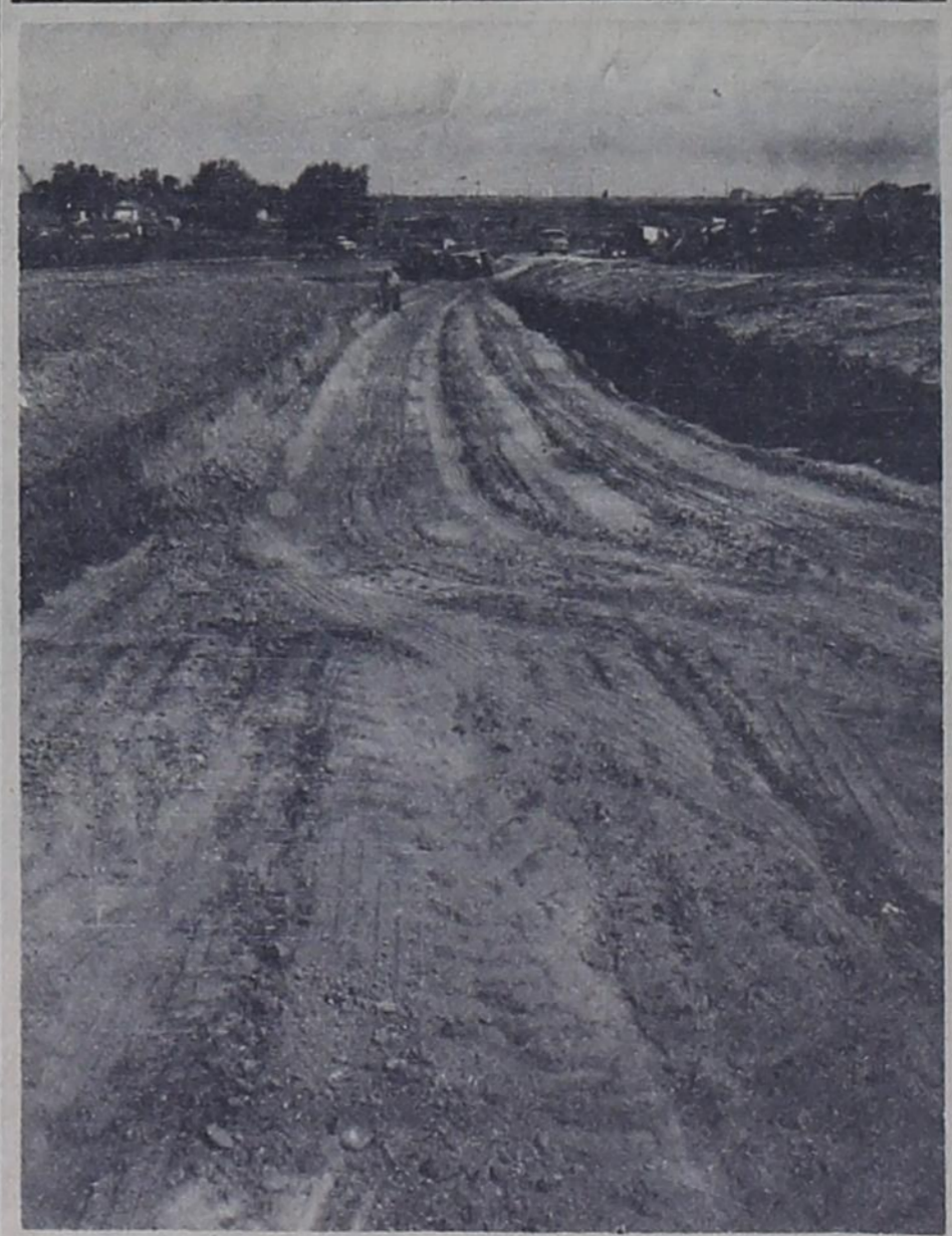
NEW PIT --- City of Bovina will soon have a new pit at the dump grounds, Contractor is Luther Vaughn of Shallowater, who is also providing pipeline ditches in Eastview Addition. The pit is expected to ease the space problem which has been facing the city dumpgrounds some time.
