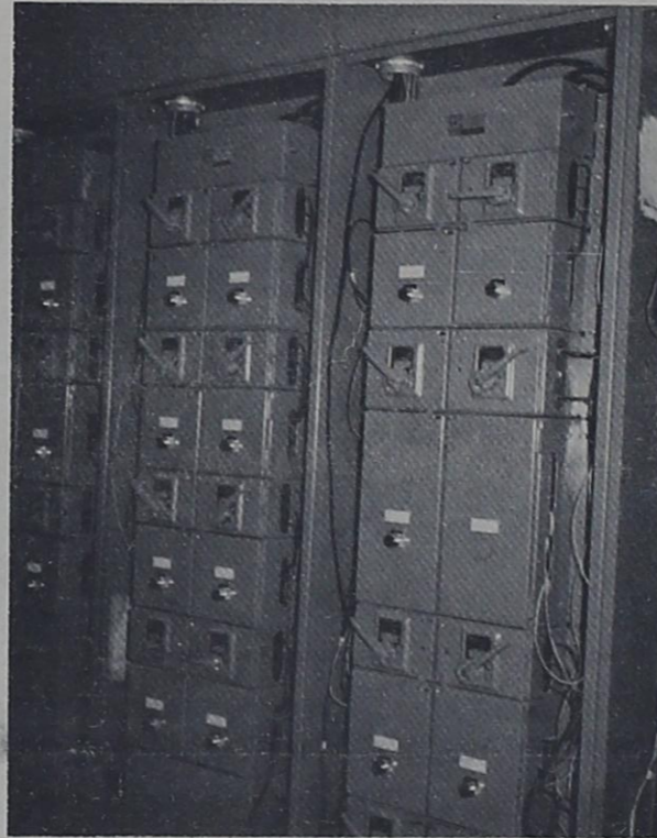
A portion of the control panels installed by Witherspoon. They are exclusive industrial electrical contractors. Bonded for each and every job.
