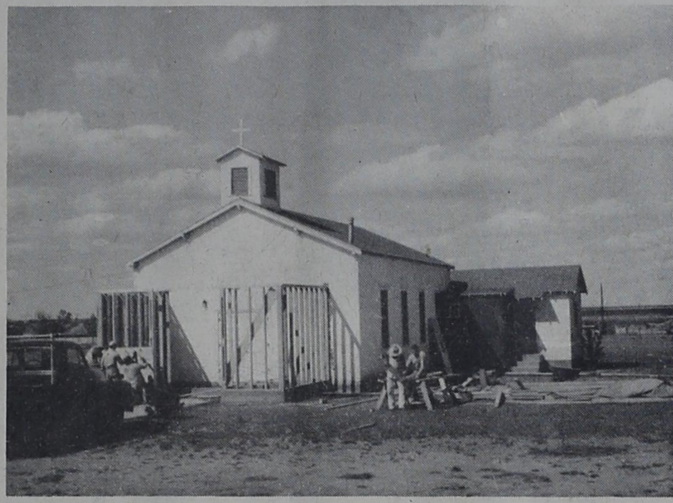
CHURCH REMODELING--Workers are busy this week making improvements to St. Ann's Catholic Church on Third Street. A new entrance is being constructed to the building to provide additional room and protection from weather. S. A. Brito is in charge of the work.
