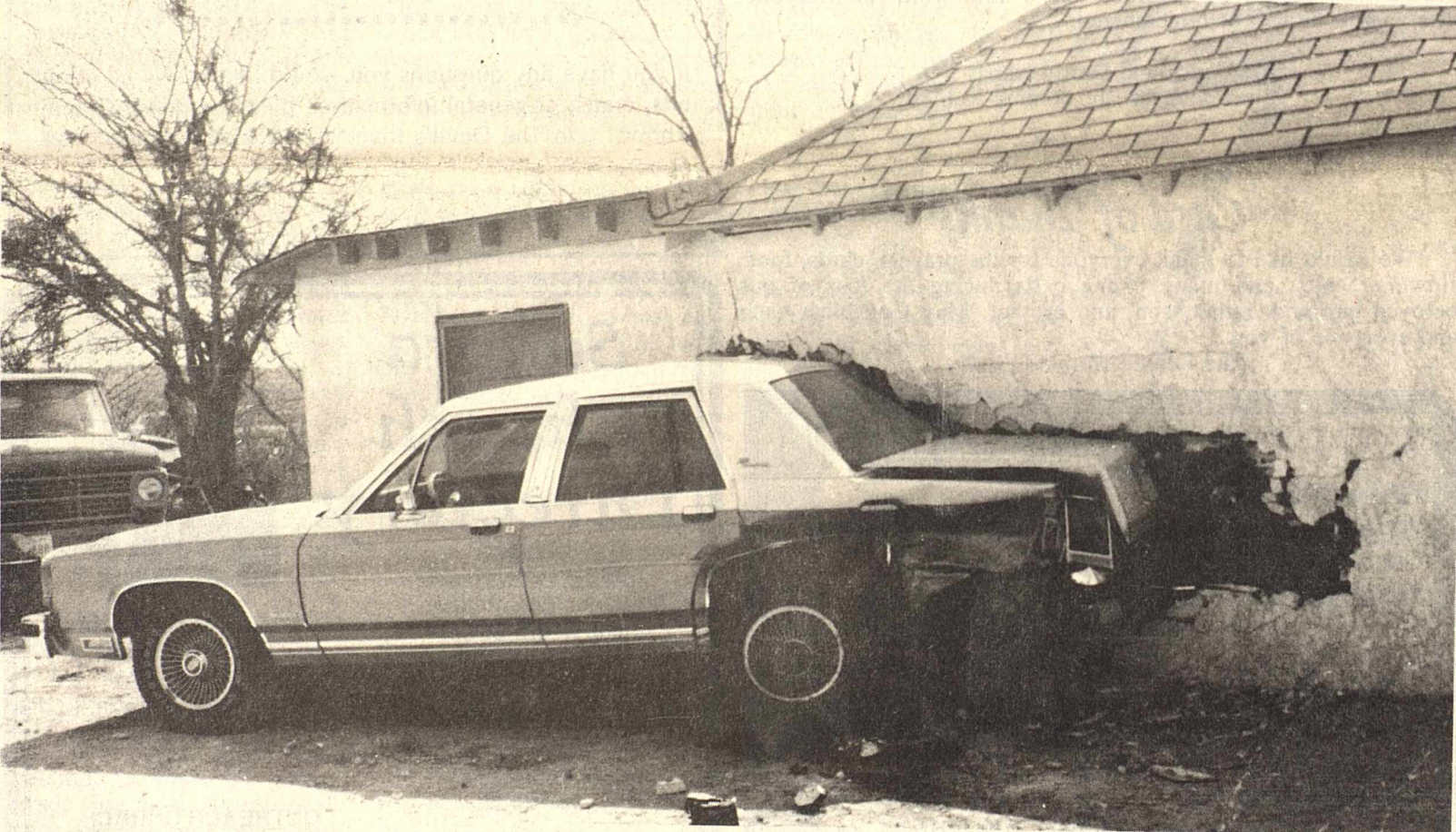
Pictured above is the aftermath of collision which occurred Friday, March 22 on St. Ann's Avenue. Estimated damage to the house is $20,000.
