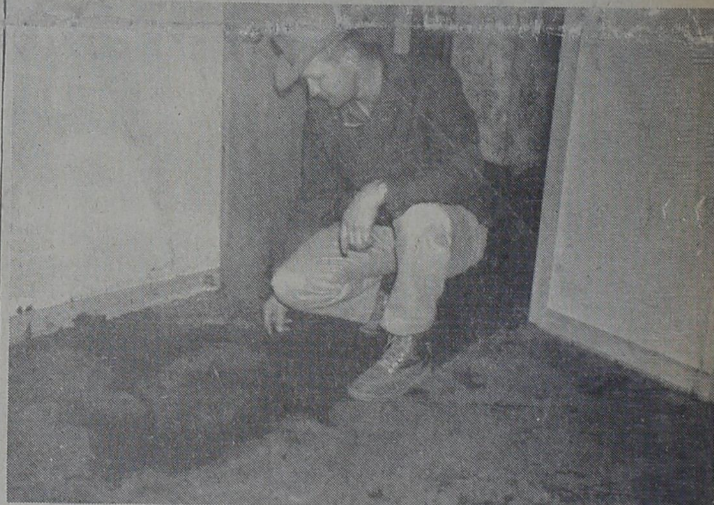
GRIM TASK -- J. D. Kirkpatrick examines damage to his house. The carpet is in a bedroom, adjacent to the bathroom where the fire originated. Behind Kirkpatrick is a trail of charred carpet where the fire worked its way to the bedroom.
