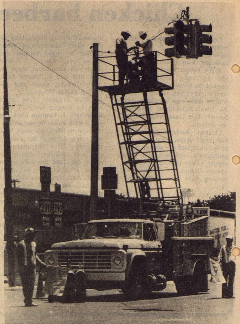
Working hard to repair the street lights on the corner of Crockett and the Del Rio highway Devil's River News/Kristi Nunn are Sutton County's Highway Department. Keep up the good work fellows.
