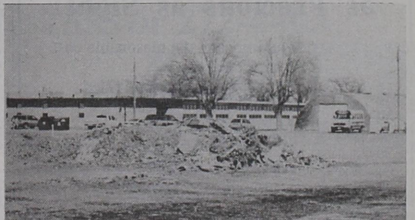
DEMOLITION... The old fieldhouse at Bovina ISD was knocked down and burned this past Monday in order to make room for the new one. The new fieldhouse will have a weight room, concession stand and restrooms. Construction will begin on March 1 by Pharr and Company of Lubbock and is set to be completed by August 1 in time for the next football season.
