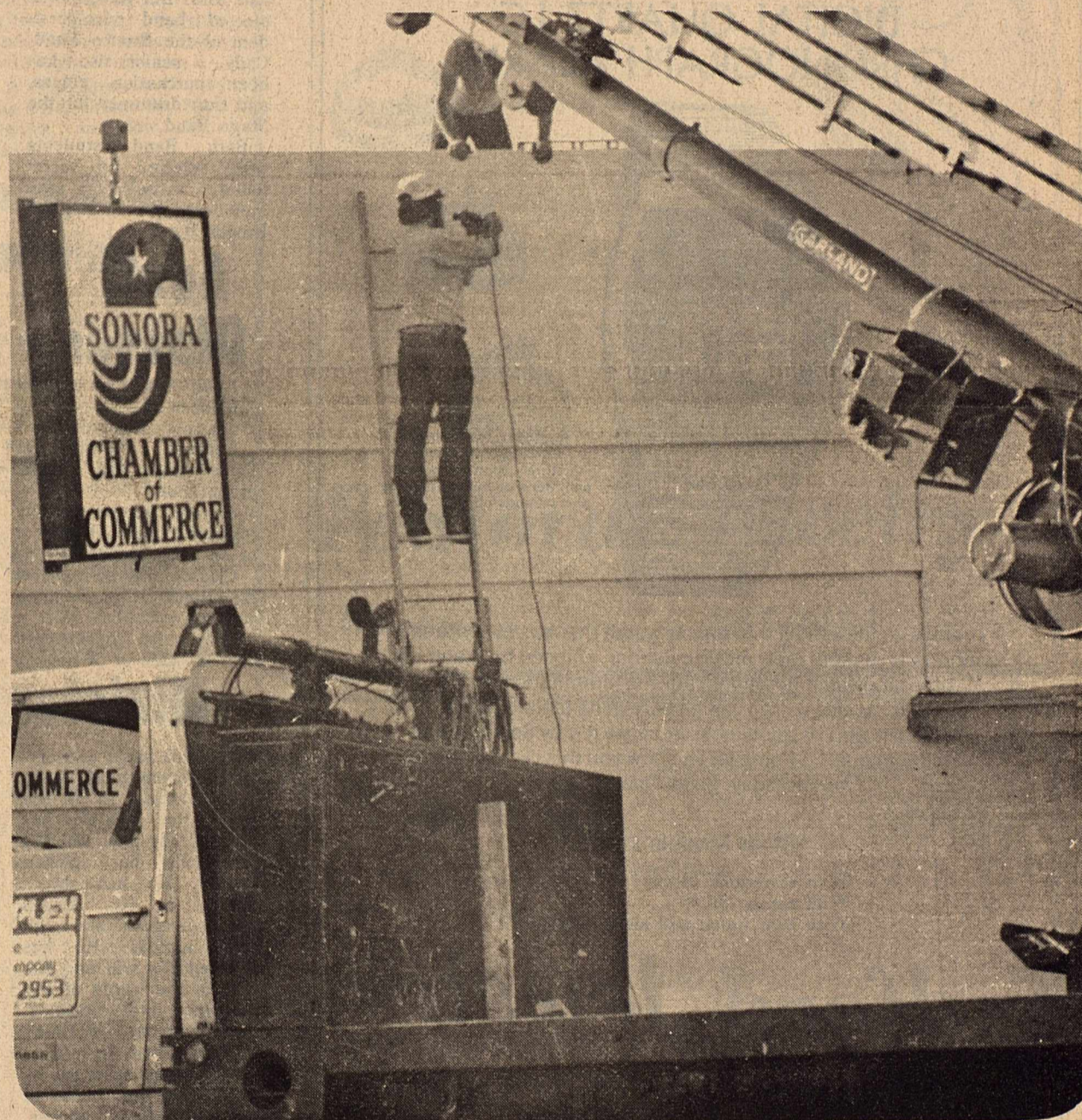
Triplex Sign Company works at hanging the new Chamber of Commerce sign downtown Friday morning.
