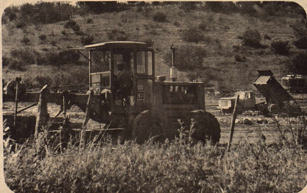
Reece Albert Construction Company of San Angelo started moving dirt on the 14-acre site for the new Halliburton Services Plant. The plant is located on
