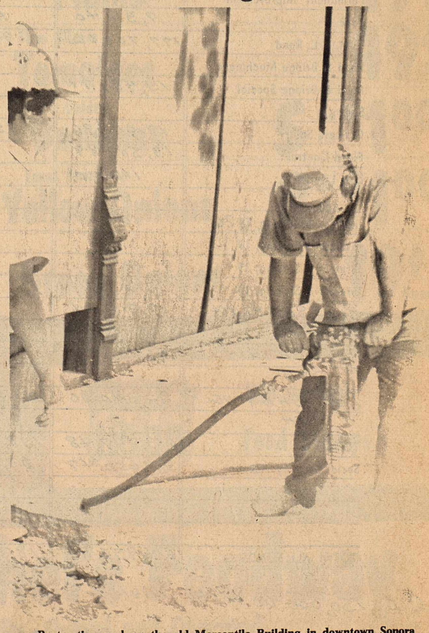
Restoration work on the old Mercantile Building in downtown Sonora continues, with concrete crews blasting away for the new parking area in front. The building is expected to be completed in a few months.
