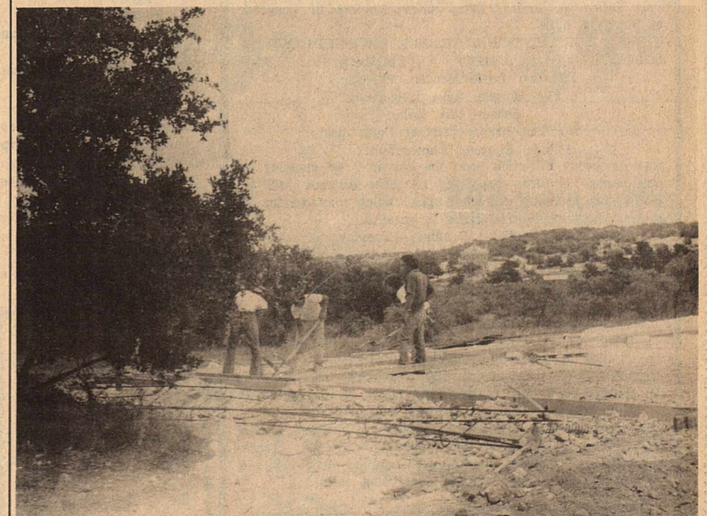
Workmen go busily about the preparation of a foundation for the doctor's clinic being built adjacent to Lillian M. Hudspeth Hospital. The 3,700 square foot building will have a brick exterior and will house two separate units. D & M Company of Del Rio is in charge of construction.
