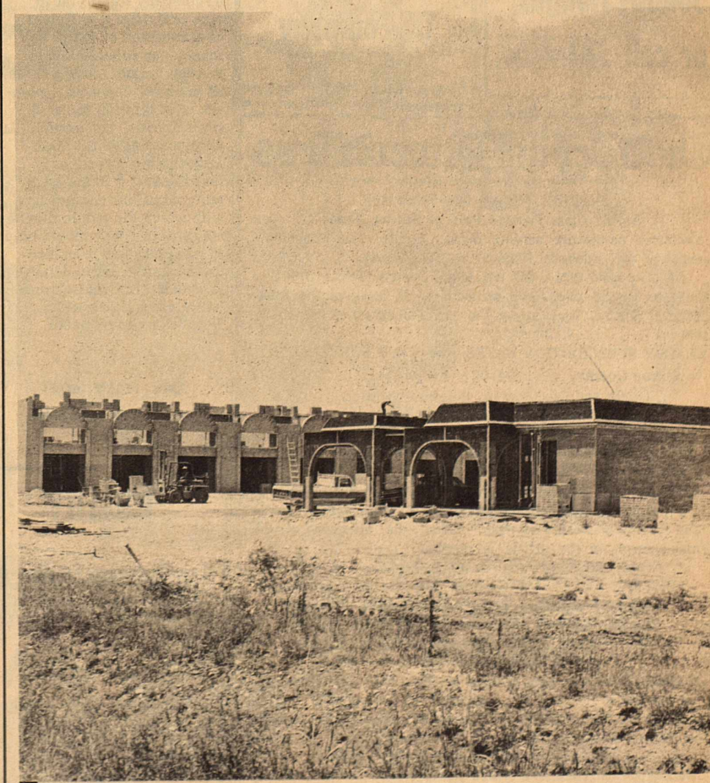
COMPLETION DATE has been set for October of the Devil's River Motor Inn, under construction on the IH-10 site near the Golf Course. Alexander Brothers Construction Company of San Angelo is in charge of construction of the motel that will feature a swimming pool. Plans for a
