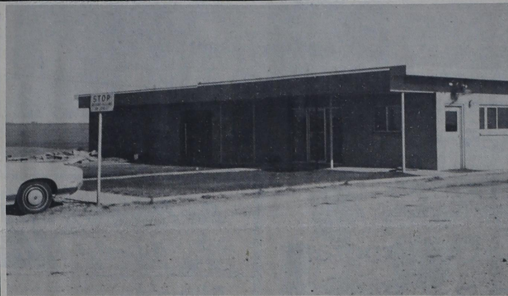
OFFICE ADDITION --- Office space at Parmer County Cattle Co. here is being expanded. Construction now underway will approximately double the amount of office space, according to
