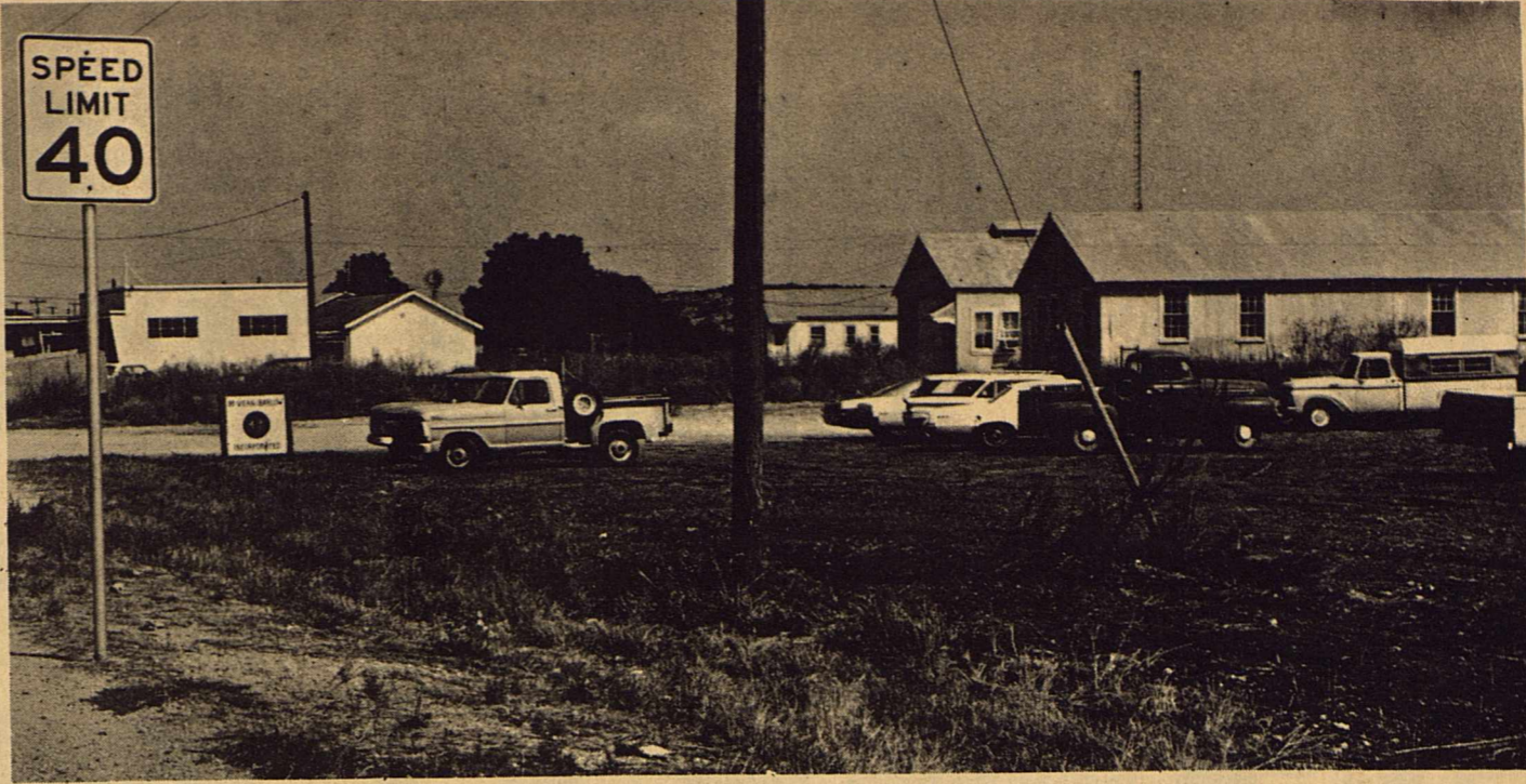
EMPLOYEES OF McVEAN BARLOW Construction Company of Odessa use this city owned property as a parking lot during their long hours in the field constructing a 36 inch pipeline in
