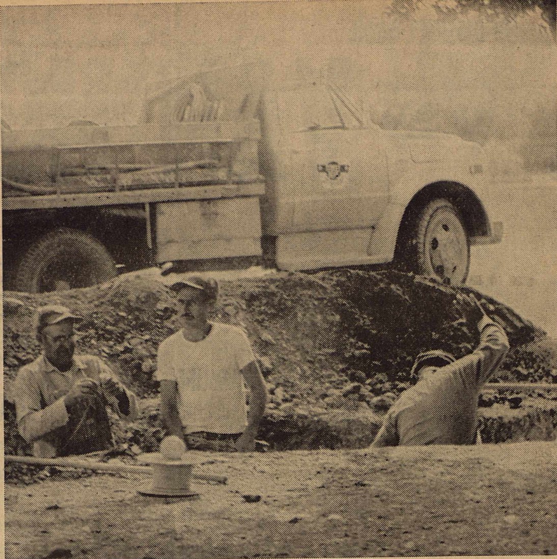
CITY EMPLOYEES (l-r) Oscar Jimenez, Sosimo Loya and Lupe Chavez are digging the ditch for the new sewer line to Loma Alto. Connecting into the city sewer system is something residents of Loma Alto have sought for a long time and now the possibility is here.
