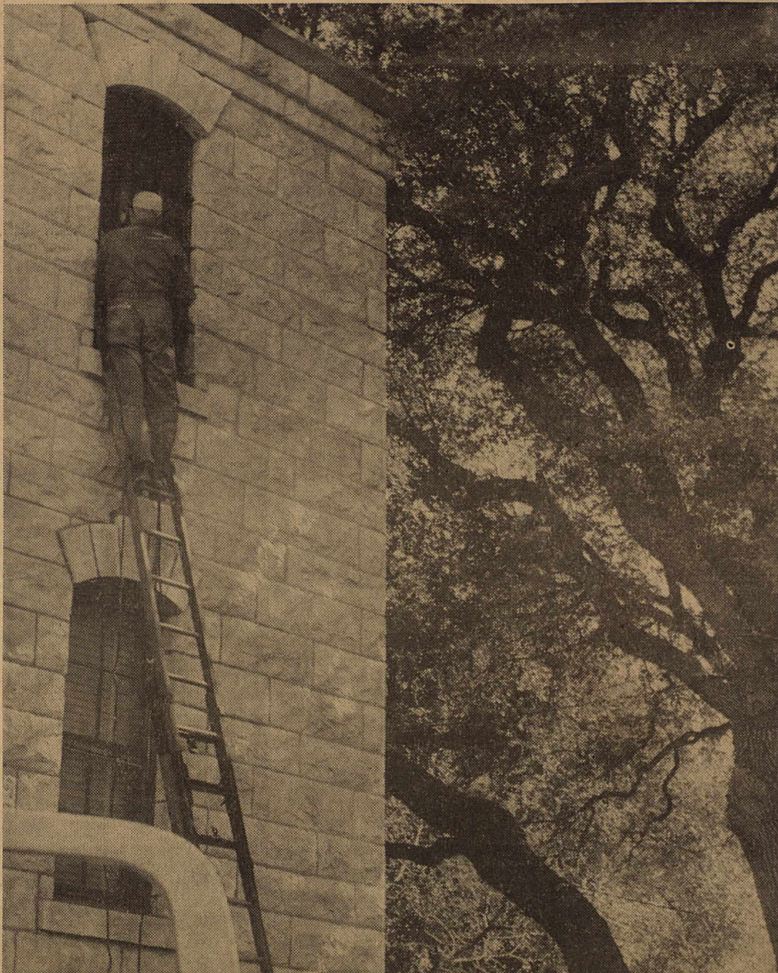
WELDING BACK THE BARS After a "Saw-out" last Thursday is this county employee. Two Mexican nationals escaped about 5:30 a.m., but a third would not flee. Bars and a heavy outside mesh screen were cut by what appeared to have been a hack saw. Antonio Rivas, 25, was under
