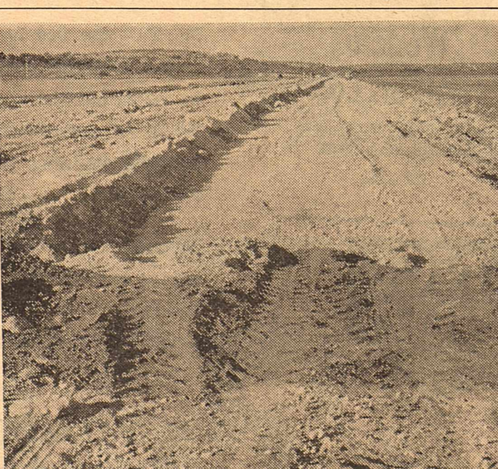
CONSTRUCTION on the new approach to the municipal airport has begun and the area has been leveled and is ready for grading. Portions of the old runway can be seen in the upper left. Construction of Interstate Highway 10 made it necessary to relocate the runway slightly from its original position.
