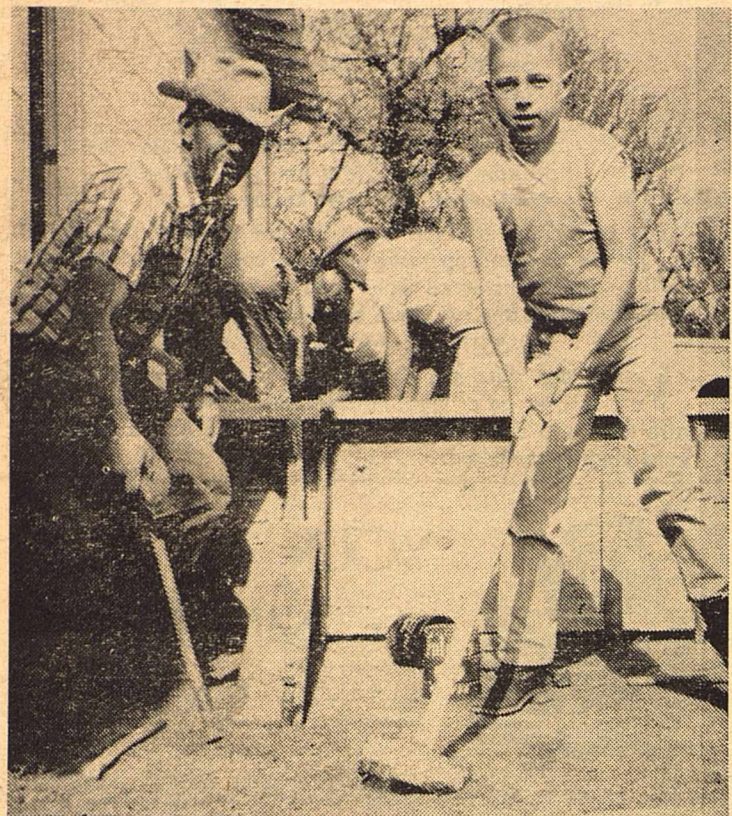
It wasn't just the men who put in their licks at the clubhouse last week. Tony Renfro joined dad Wallas in driving stakes as concrete forms were set up for the new walks, steps and patio. And Tony knows the difference between a golf grip and a sledge grip!
