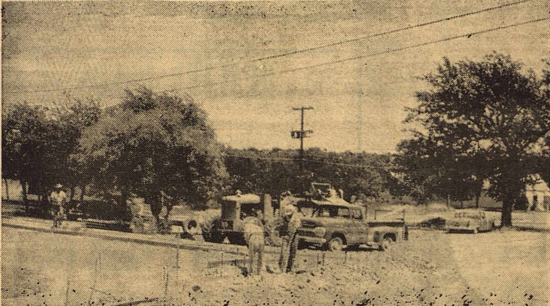
City employees are pictured here as curb and gutter work was underway on Lomax Park. The City plans to improve the park, a triangular shaped lot about an acre in size donated to the city about a year ago.
