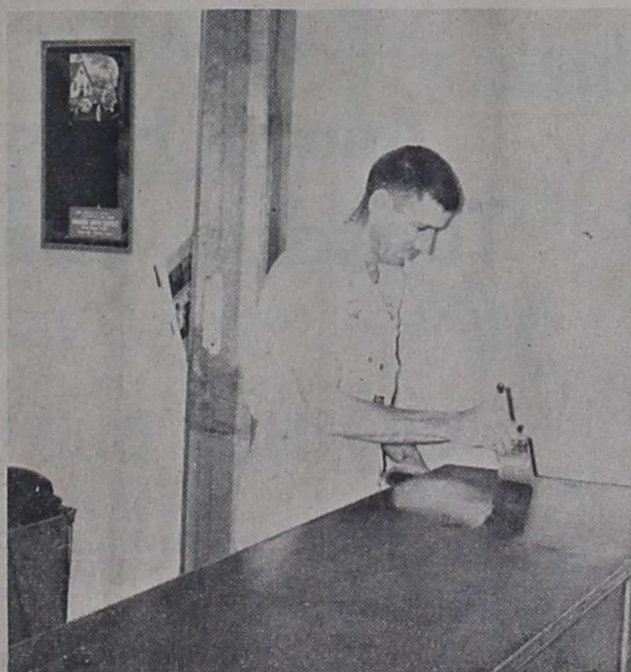
NEW PAINT--Glenn Hromas, paint contractor here, is shown applying a coat of varnish to a counter in city hall. This was a part of the repair work done on the city-owned property during past several days. The building received new paint and varnish inside and out and a new ceiling was installed in city hall portion of the building. Work was done on Saturday afternoons and nights so as not to interfere with regular city business.
