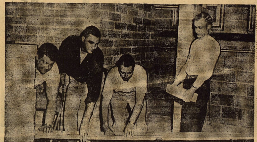
JAYCEE SHELTER project, part of the organization's nationwide "Operation Survival," takes concrete form as Blue Earth, Minn., Jaycees construct a 4-person fallout shelter in the city hall basement. This is one of a variety of permanent or temporary display shelters built by Jaycees in cooperation with civil defense in communities across the nation. Each of the 3,900 Jaycee chapters in the United States is being encouraged to participate in the program to stir public interest in fallout shelter construction in every community across the Nation. (Fairmont, Minn., Sentinel Photo)
