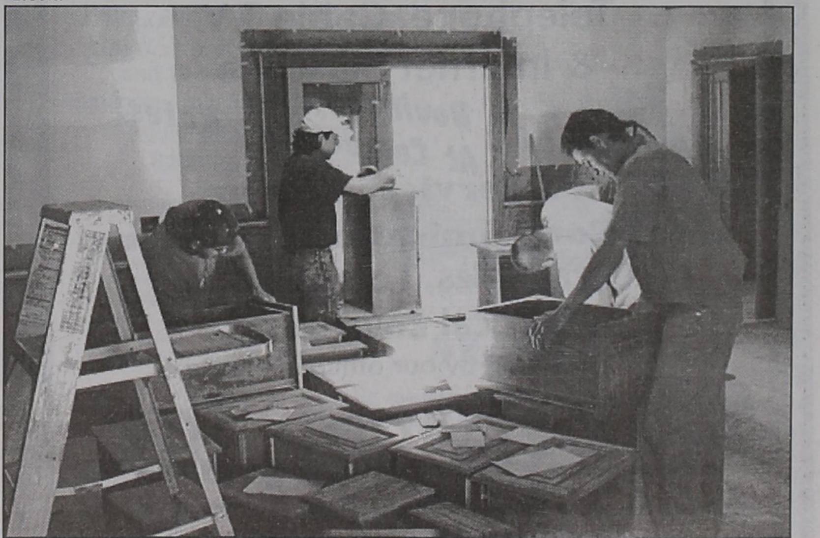
and finishing the inside cabinet work. The best estimate is the building will be ready for occupancy by September. ron carr photos
